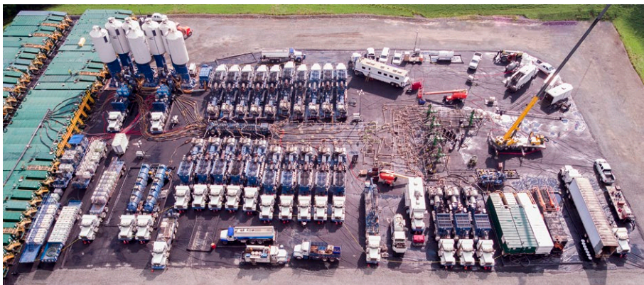
Figure 1: Typical hydraulic fracturing fleet with 23 diesel powered fracturing pumps and support equipment
